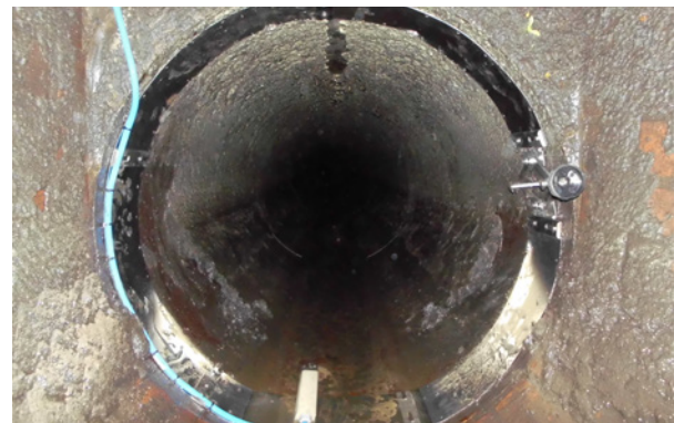
Installed Nivu probes in the Rodenkirchen sewer network. © Nivus GmbH
