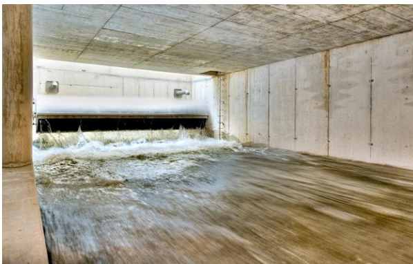
Controllable stormwater holding tank. © StEB Köln
